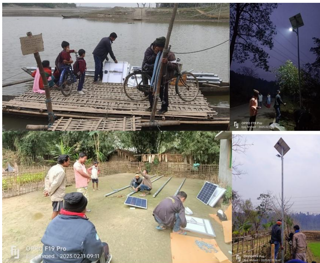
Figure 11. Solar-street lights transportation, and installation at strategic locations in villages which can minimise accidental encounters with wildlife by increasing the visibility in the area.
